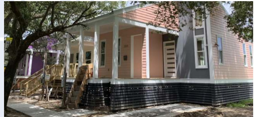
Ongoing construction of new affordable housing on Andry Street - LOWER NINTH WARD
